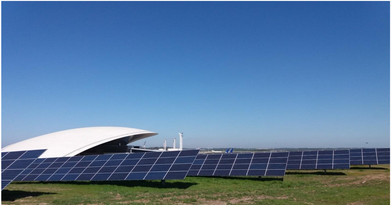
Solar Photovoltaic Plant
